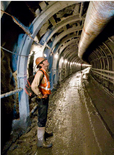
Figure 1. Shawn Spreng Examining Outlet Tunnel Ventilation Pipe; Lenihan Dam Outlet Modification Project, Los Gatos, California, USA
